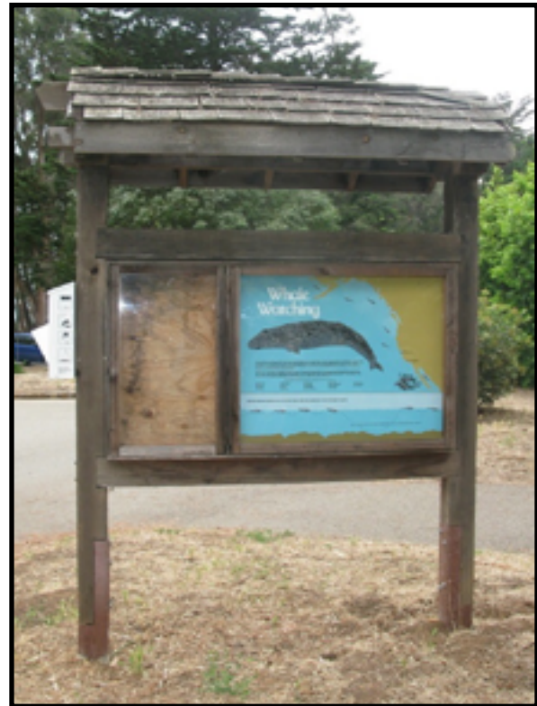
Figure 25. partially empty panel shelter
